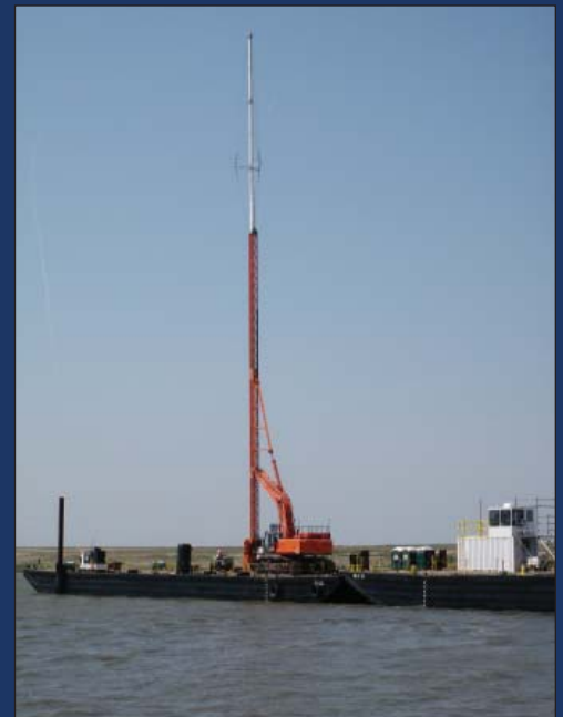
The excavator driving on top of the barge inserts the wick drains by drilling through the dike's sand lifts with a 160-foot long steel mandrel.
