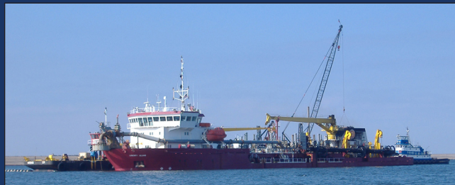
The Liberty Island hopper dredge is assisted by several tugboats while taking its position in the harbor to transfer sand to the spill barge.
