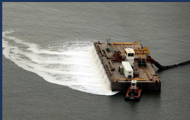
Great Lakes Dredge & Dock's specially-designed spill barge distributes layers of sand onto the footprints of the south and division cross dikes.
