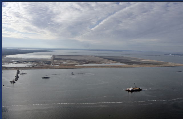
An aerial shot of the project location shows the existing Craney Island in the background and the location of the eastward expansion in the foreground. The expansion will add 522 acres to the east side of Craney Island.
