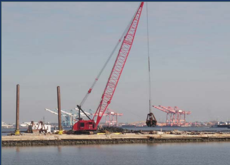
GLDD subcontractor WF Magann is finished demolishing the outer 300 feet of the rock jetty. More than 10,000 tons of debris has been removed.
