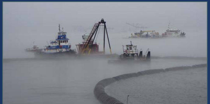
Even with heavy fog on the river, tugboats position the floating pipe for the next load of sand.
