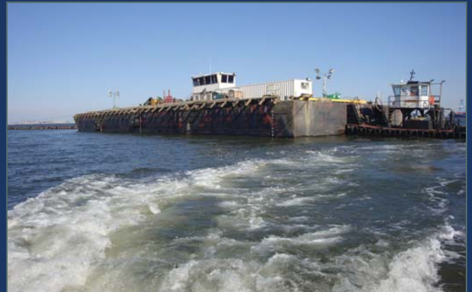
The spill barge prepares to send another load of sand onto the dike footprint.
