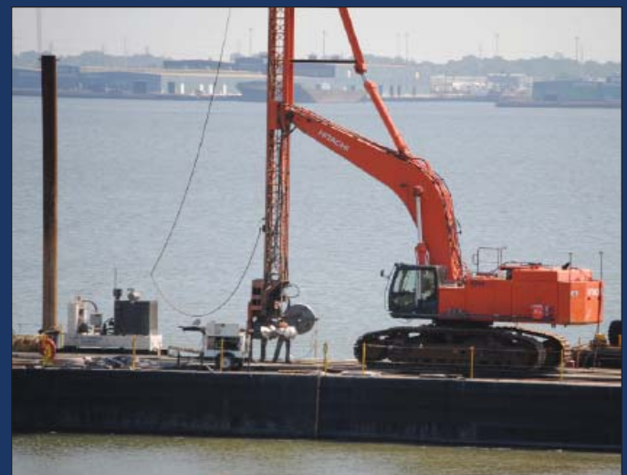
Wick drain installation for Stage 2, shown above during Stage 1, will be awarded in a separate contract from the sand placement.
