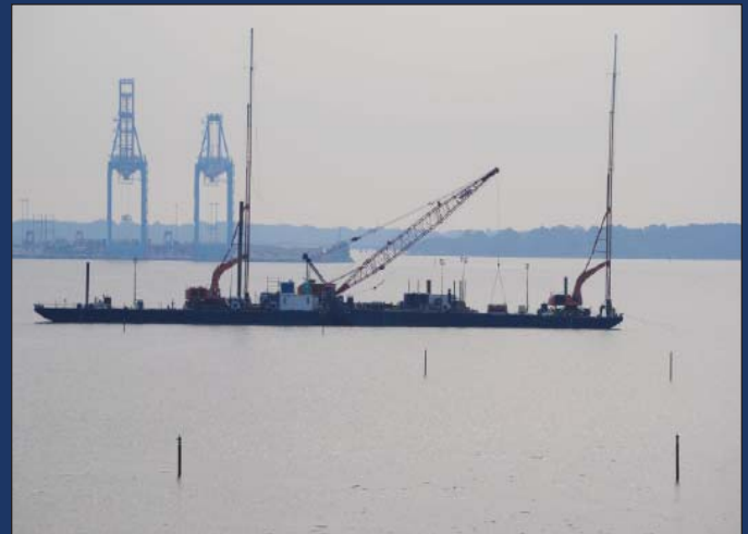
After late August's earthquake and Hurricane Irene, USACE Project Engineers inspected the existing CIDMMA to verify the facility was not damaged. Ongoing construction at CIEE is monitored by periodic surveys and instrumentation (the pipes in the water above).
