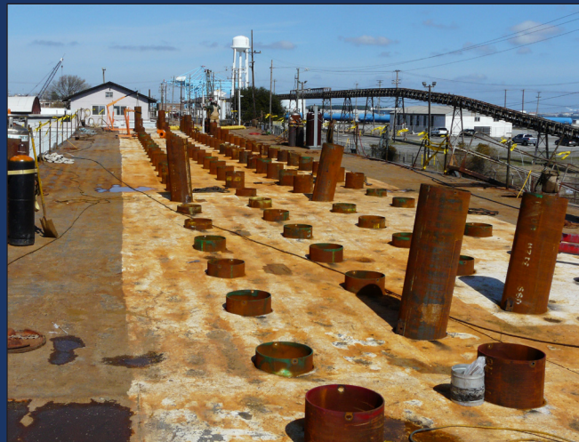
The barge being used for installing the PVDs is being fabricated at W.F. Magann Corporation's facility in Portsmouth. These holes with pipe sleeves installed in the deck will make wick drain placement more efficient.
