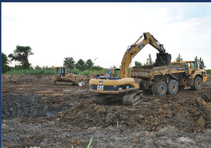
Using large excavators and off-the-road trucks to move dirt at the site maximizes project efficiency.
