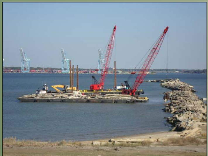
W.F. Magann Corporation is in the process of demolishing the outer 300 ft. of the rock jetty at Craney Island. Norfolk International Terminals (NIT) can be seen in the background.
