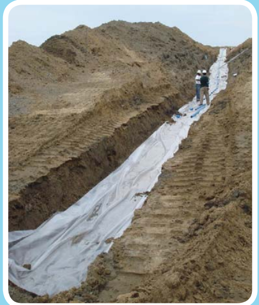
A Horizontal Inclinometer was Installed In A Trench To Measure the Settlement Profile of the Berm
